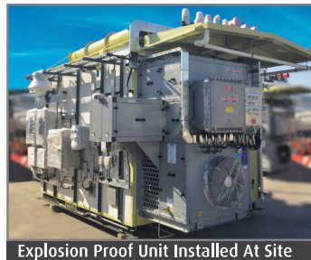
Explosion Proof Unit Installed At Site
