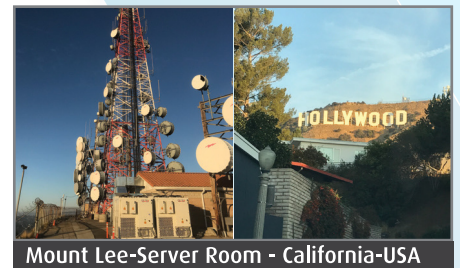
Mount Lee-Server Room - California-USA
