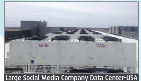
Large Social Media Company Data Center-USA
